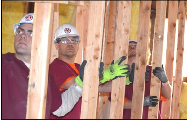
AGC Graduates place a new wall into position at their project house on East 31st Avenue. The house was heavily damaged by an arsonist and it's reconstruction is being organized by Habitat For Humanities.
